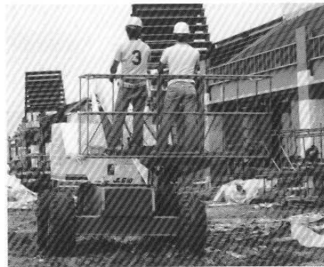
Optional oscillating axle and four wheel drive combination provide the means to negotiate demanding conditions.
